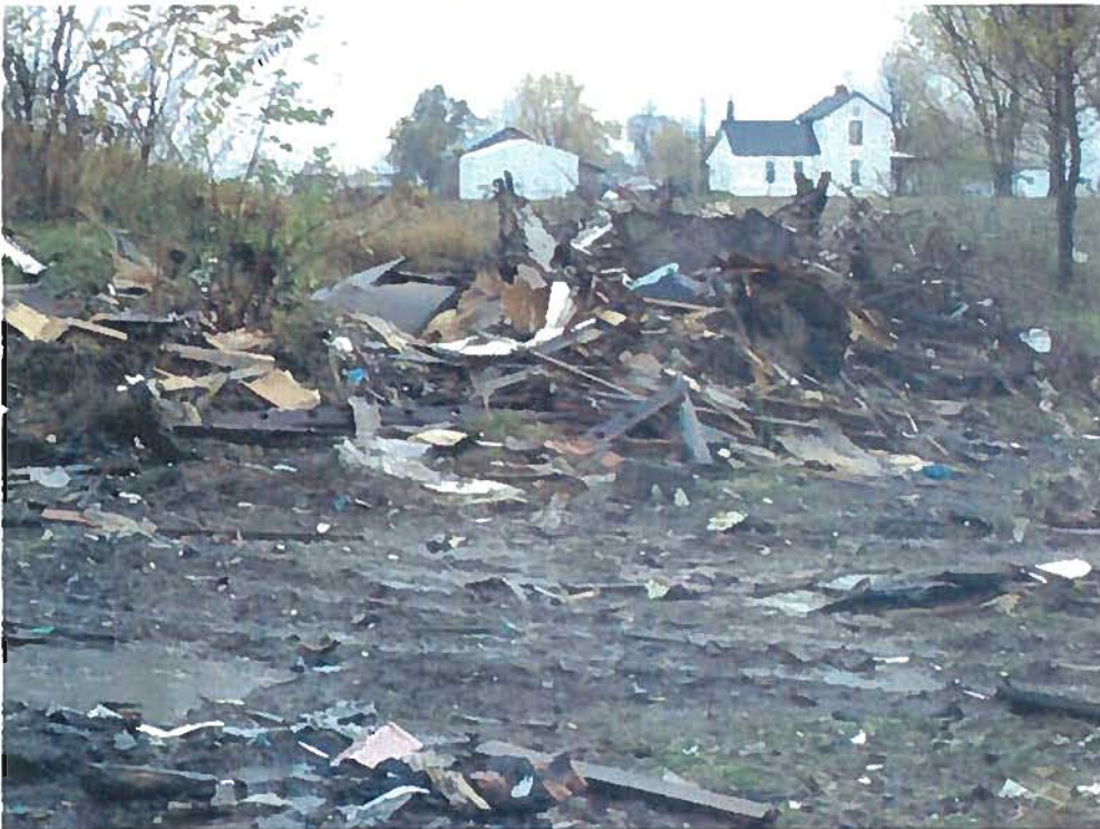
Date: November 3, 2011 Time: 12:38 p.m. Direction: E Photo by: Charlie King Exposure #: 010 Comments: Wastes measuring approximately 30' x 15' x 5' at the location of the old open dump pile observed during the Initial site inspection on June 29, 2011.
